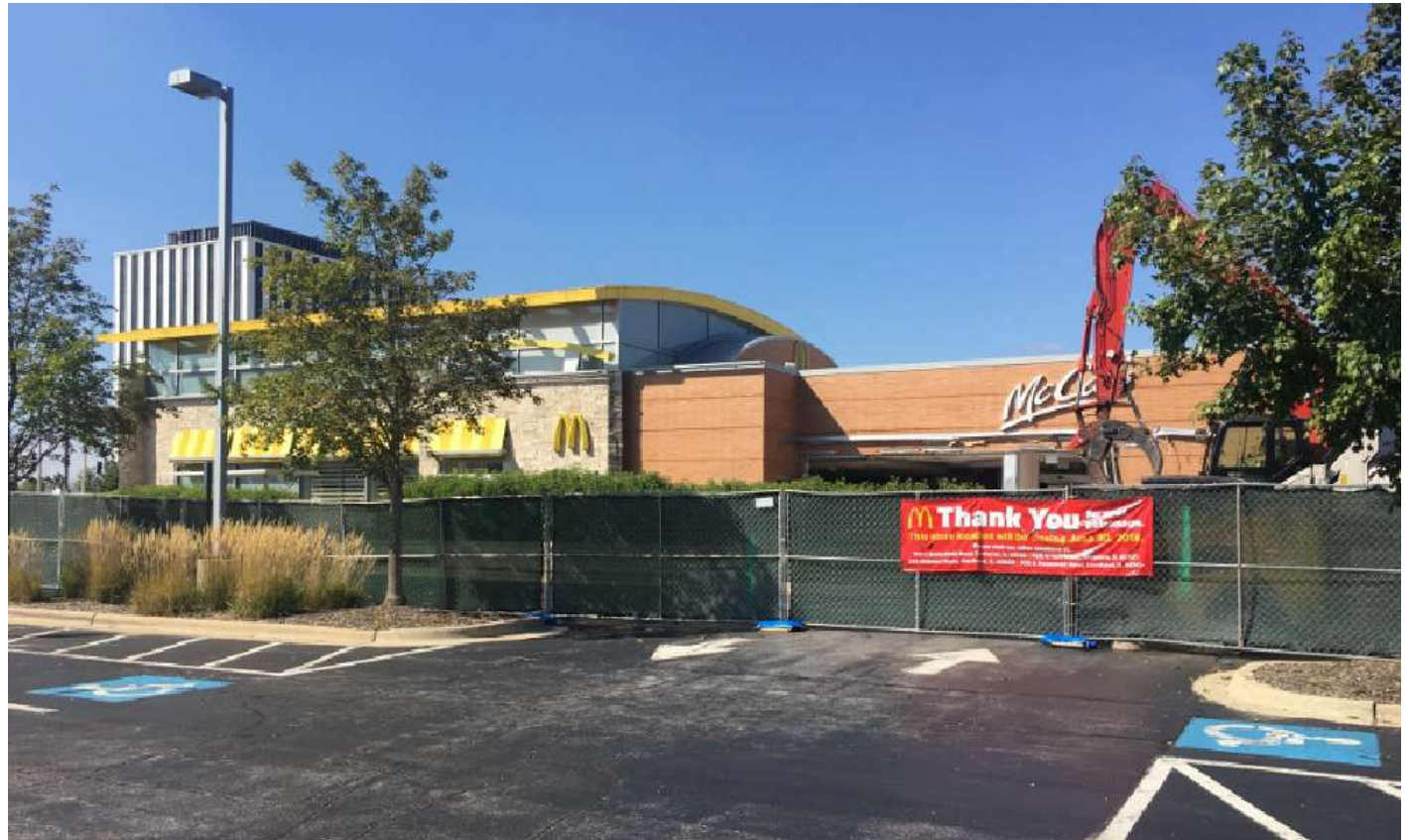
Following McDonald's relocation of its headquarters to Chicago's West Loop, a demolition crew tore down the restaurant next to McDonald's Plaza in Oak Brook. Developers and city planners are discussing the opportunities to reinvigorate the commercial district.
